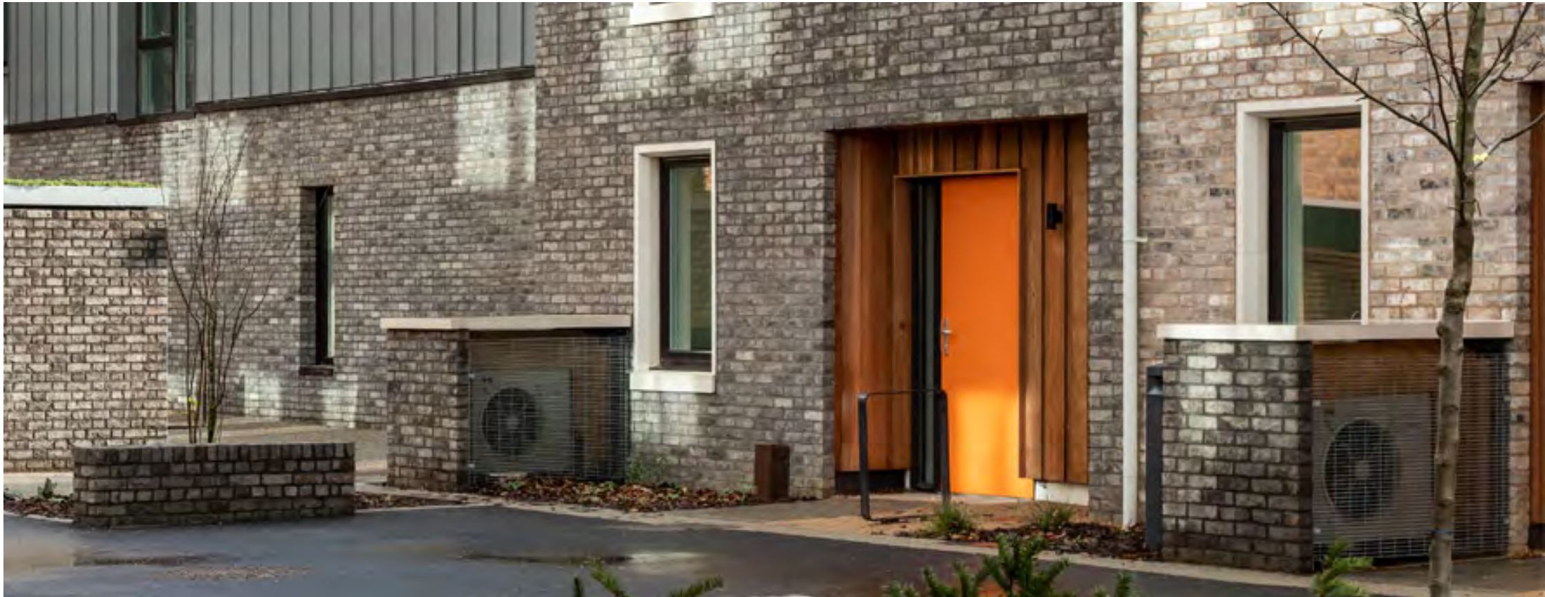
Figure 57. Air Source Heat Pumps
